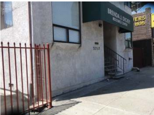
Guideline 6.1: Ground floor stucco collects dirt and is easily stained.
