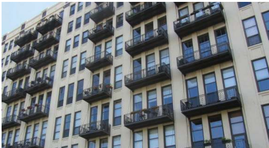
◀ Guideline 5.4.4: These balconies appear “tacked on” and not integral to the design of the building.
