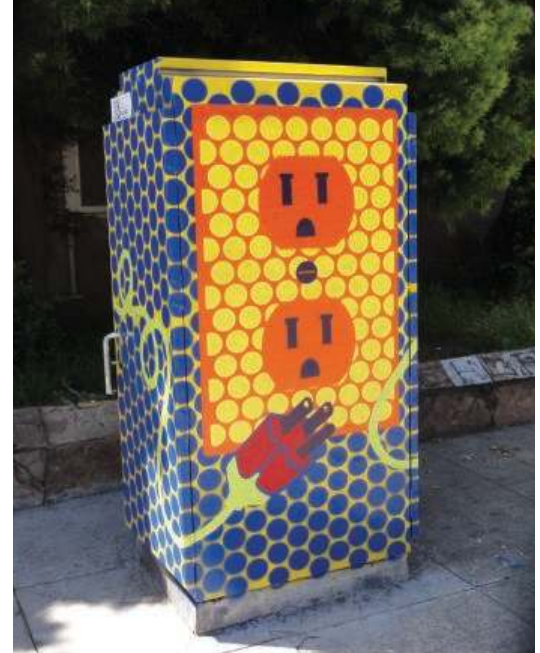
Guideline 3.3.3: Incorporate art into existing utility boxes. Place new utility boxes underground if possible.
